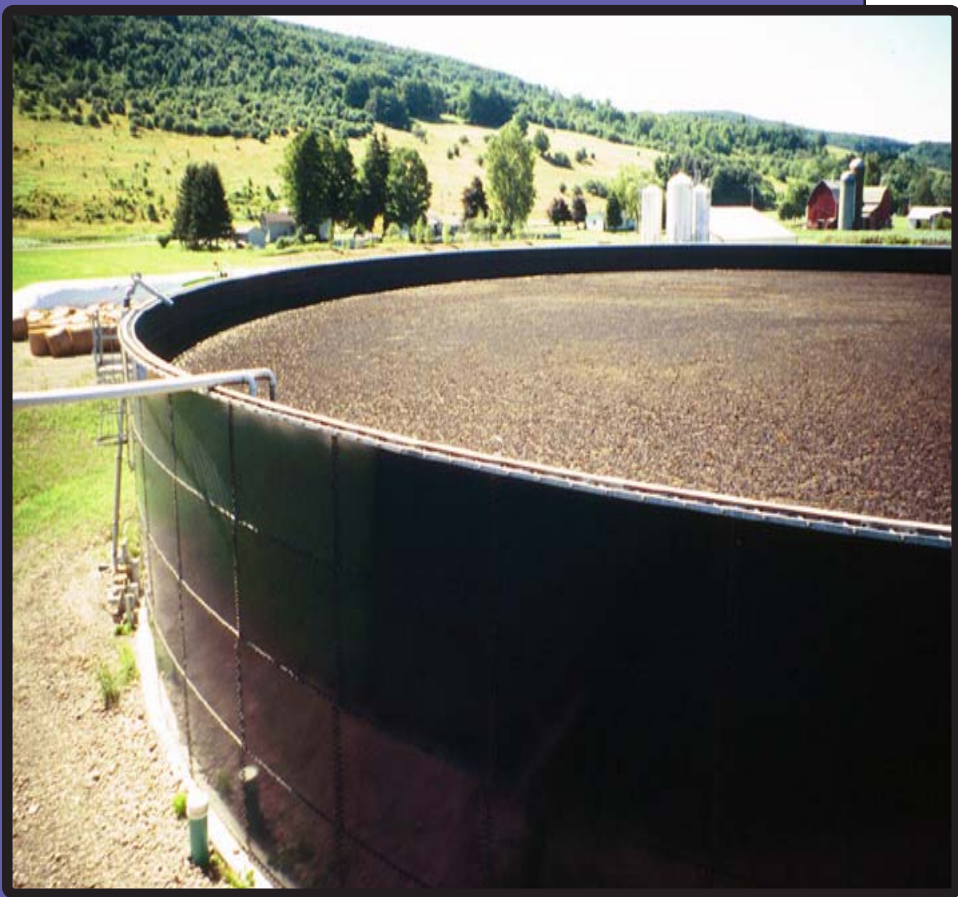
After digestion, effluent is transferred to a 2.9 million gallon storage tank
