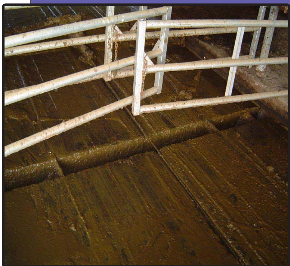
Alley scrapers deposit manure to central drops in freestall barns
