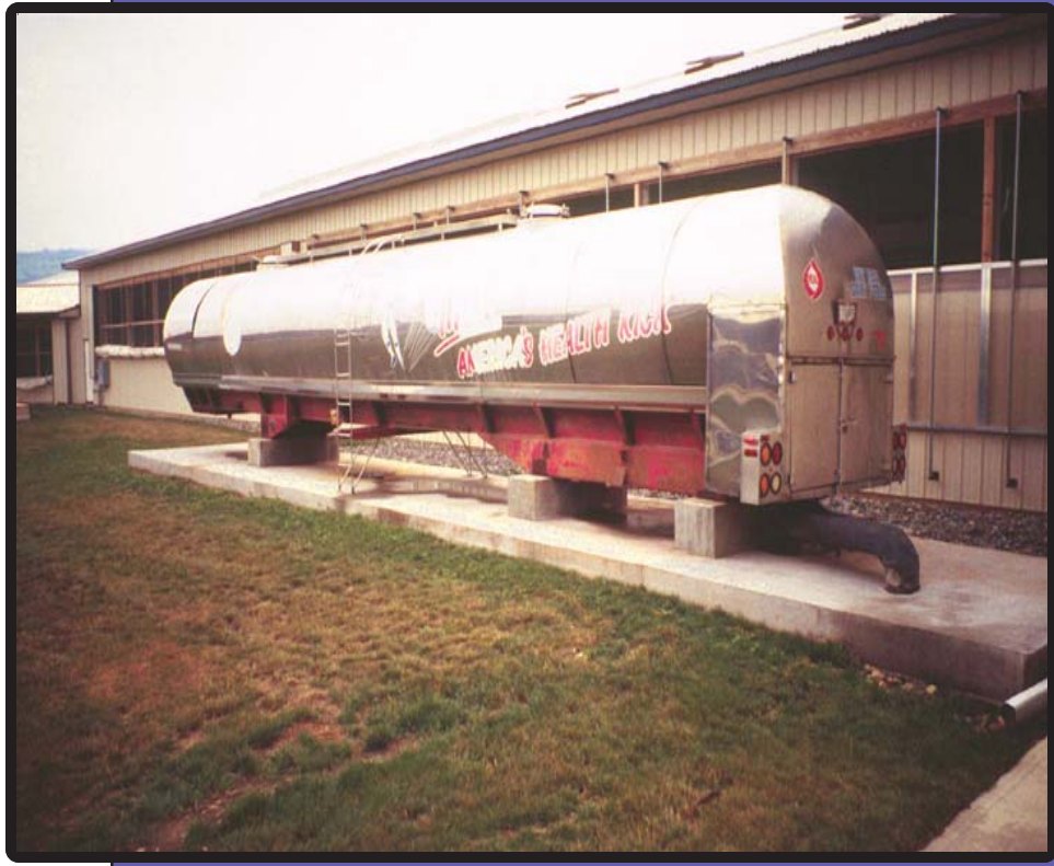
6,000 gallon hot water storage tank
