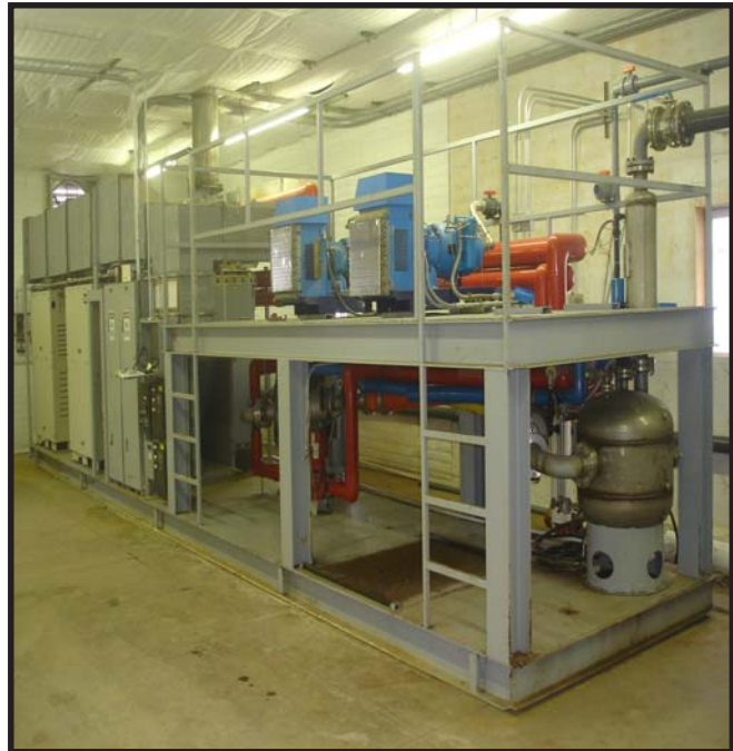
Above: De-watering and compressor equipment in foreground; Capstone microturbines in background
